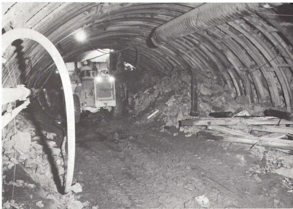
Early stages of work on the Melbourne underground rail loop. Victorian Railways Board
